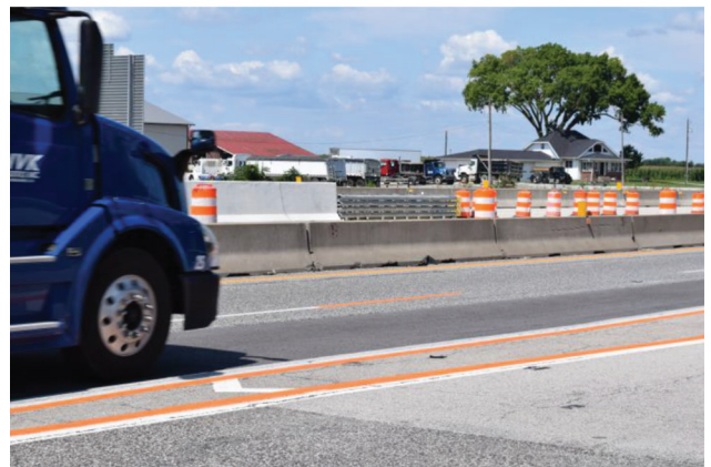
Figure 6.10 Lead/lag and complementary orange marking.
