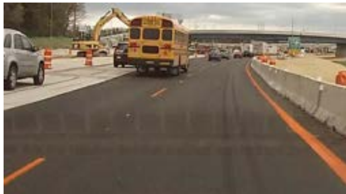
Figure 5. Orange Temporary Marking on Asphalt Surface
