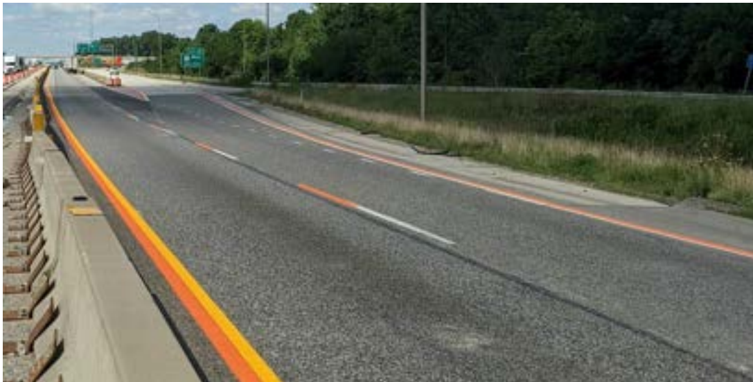
Figure 6. Supplemental Orange Markings on Interstate 65 Northbound
